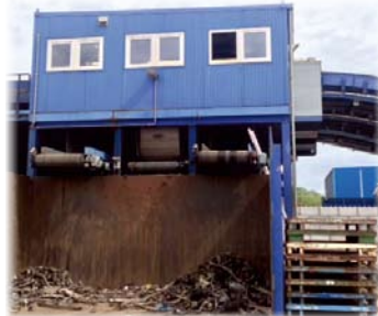
Ventilation & Venting for Sorting Cabins
